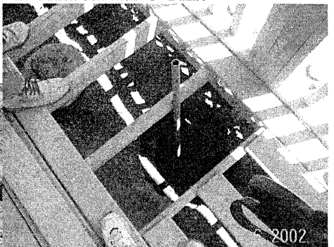
Old septic tank under front deck pipe sticking out of Hole in bottom of tank (will be filled)
